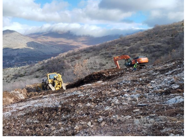
Picture 12: D9 Dozer making light work of Clearing and Grubbing & topsoil removal at BP6
