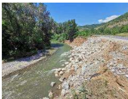
Figure 47 Lateral erosion of the Lepenec river with collapse of the river bank near the existing road
