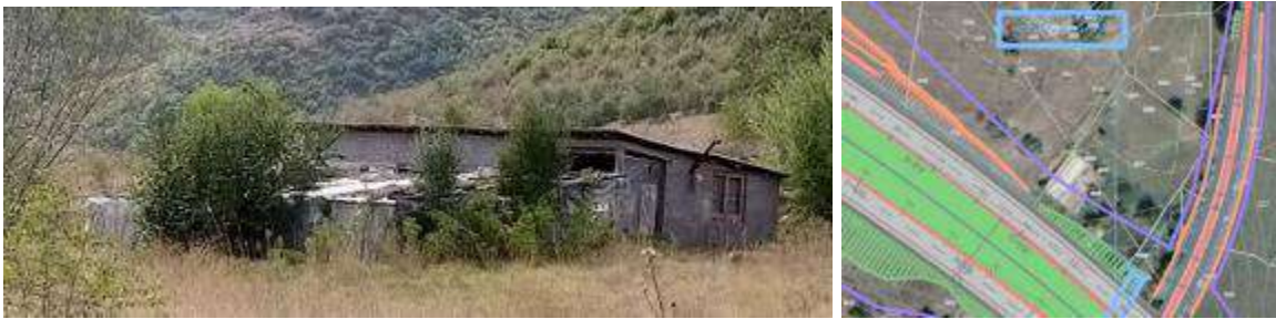
Figure 151 Improvised weekend house to be acquired and dismantled at the location I (see chapter 3.5.5)
