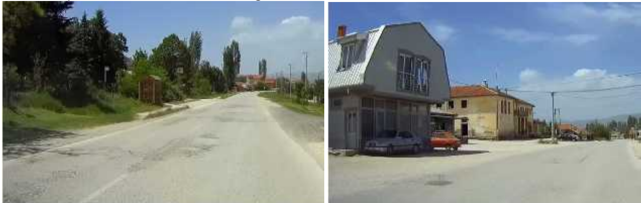
Figure 2 Beginning of existing sidewalk on left side in settlement Kukurecani - Gap in existing sidewalk
