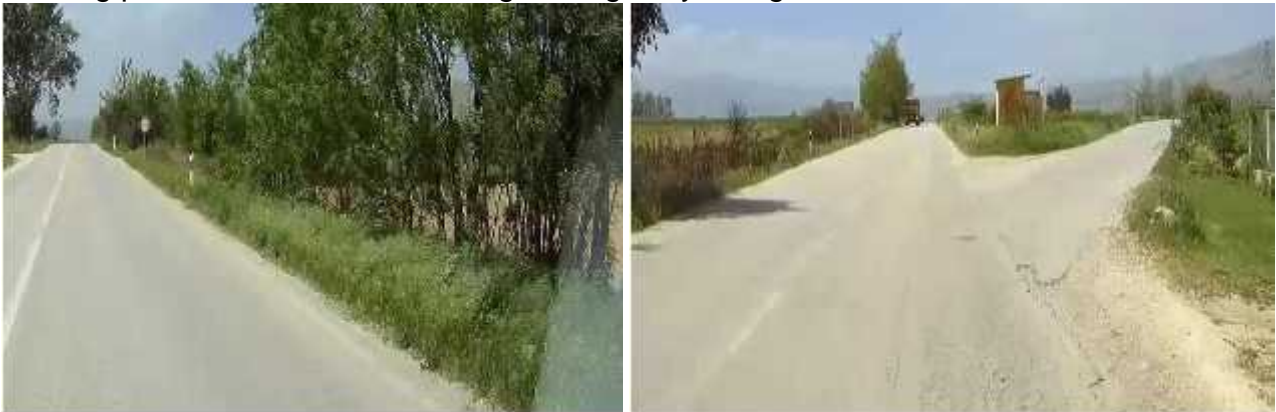
Figure 4 Unmaintained shoulder could cause water retention on carriageway- Intersection for settlement Crnobuki at km 3+623
