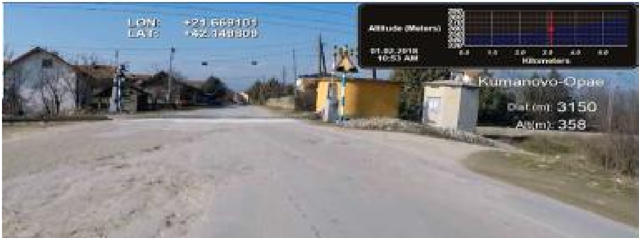
Figure 5 - passage through the railway and the damaged carriageway in this part of the road is significant and danger for the traffic safety, especially at night. Inadequate deviation of the road in front of the railway itself.
