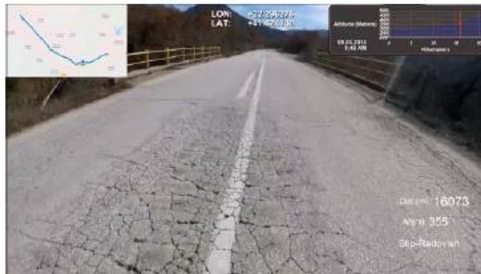
Figure 5 Bridges on the respective section are without an adequate system for retaining and protection
