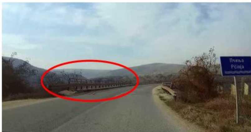
Figure 5 - Guardrail - insufficient lengths, wrong type of guardrail
