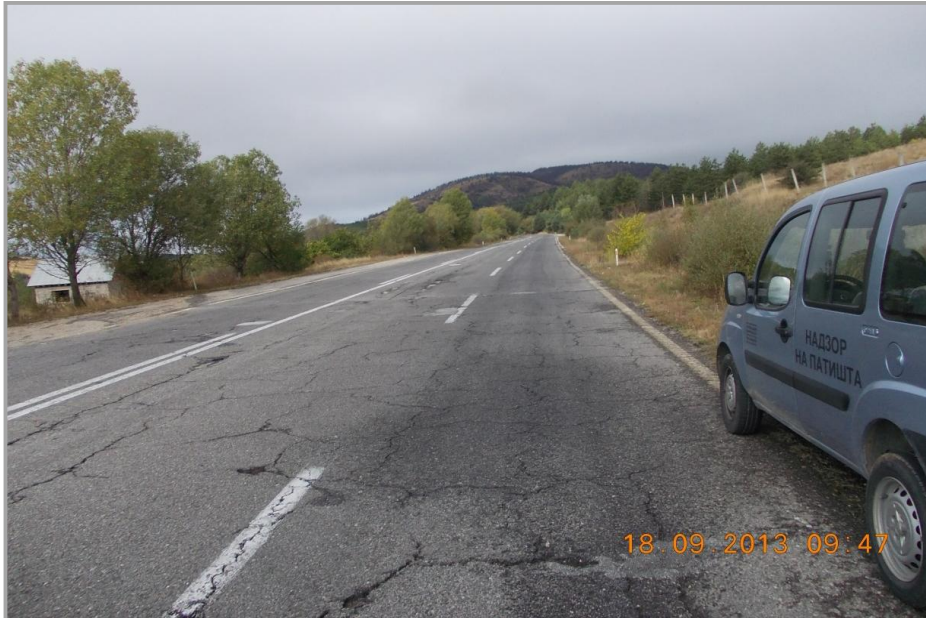
Figure 2 Damages of the pavement construction
